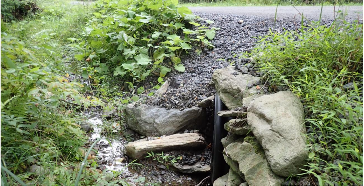
Photo 7: The roadside and culvert at 648 East Street showing overflow from road material into the swale and the collapsing structure around the renovated culvert.
