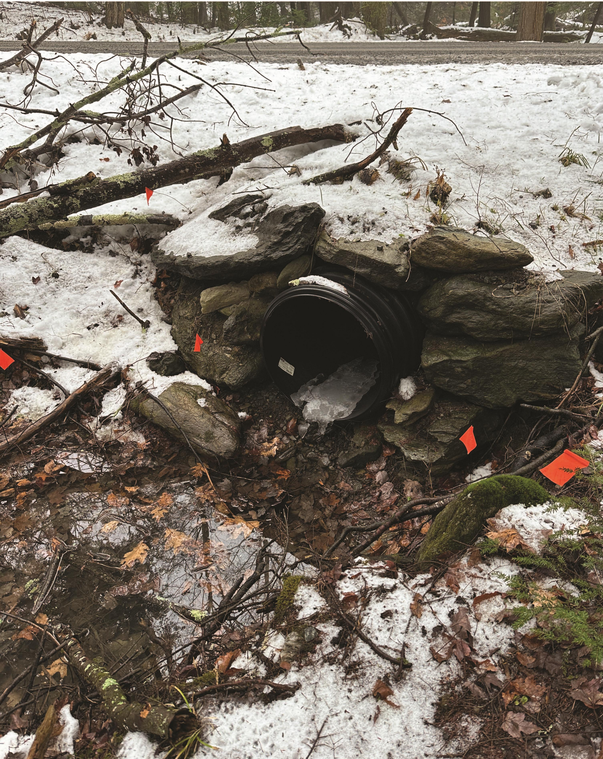
EXISTING CONDITION: NO OUTLET PROTECTION
